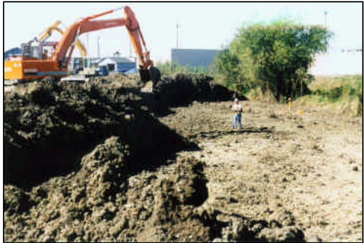
Excavating at Amazon Creek: Sept. 2001- Thousands of cubic yards of soil were removed along the creek. The floodplain was then re-contoured to create several high flow channels adjacent to the main channel.
