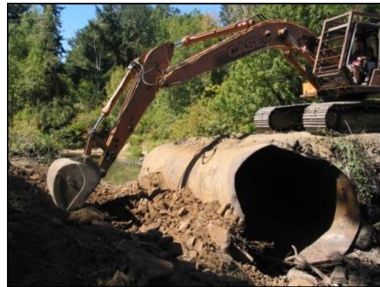
An excavator removes the undersized culvert that blocked fish passage to 46 miles of upstream habitat.
