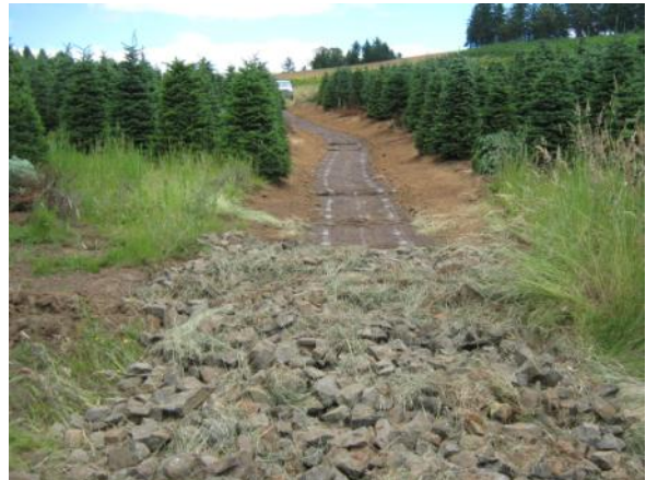
Post-project: view from bottom of drainage looking uphill. This shows the last constructed portion of the grassed waterway, that was completed in June 2010. The bottom of the drainage has a small rock pad that dissipates energy from the sub-surface drain pipe that day lights here.
