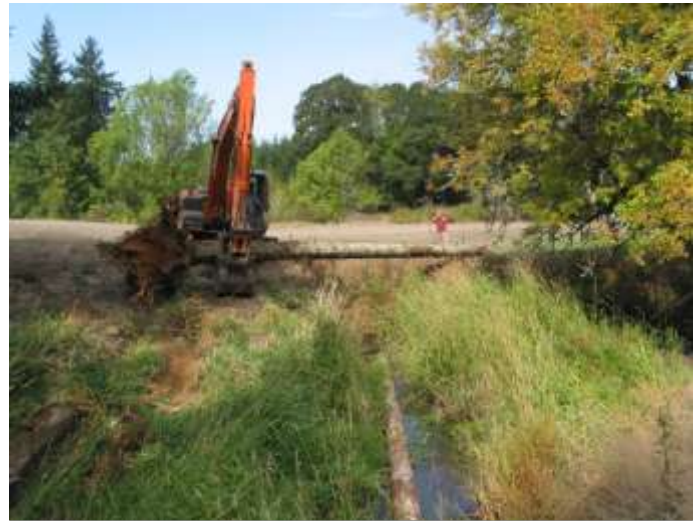
An excavator places logs with rootwads in Owens Creek to provide habitat for cutthroat trout and other native aquatic species.
