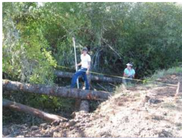
Implementation: Large conifer logs with rootwads were positioned in the tributary channel. In addition to enhancing habitat, these logs will help the channel's flow to naturally meander.
