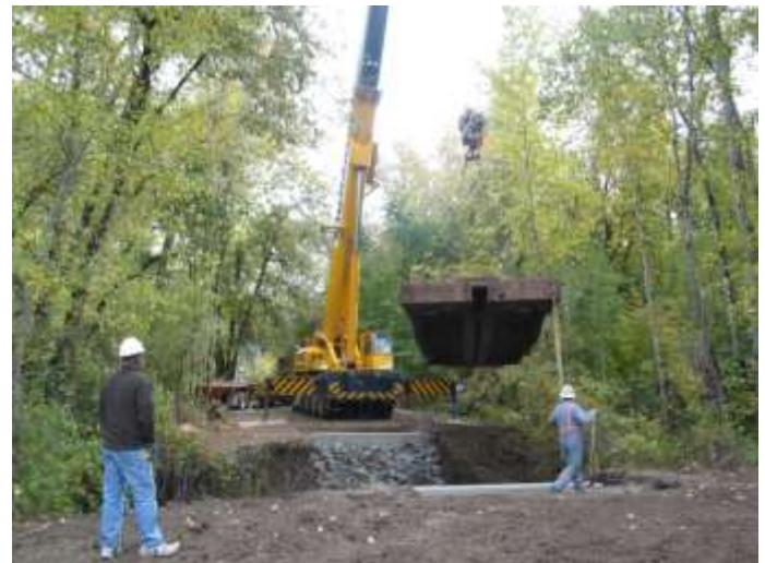
A crane places a railcar bridge over the tributary to Spencer Creek to allow the landowners maintenance access the property on the west side of the tributary.
