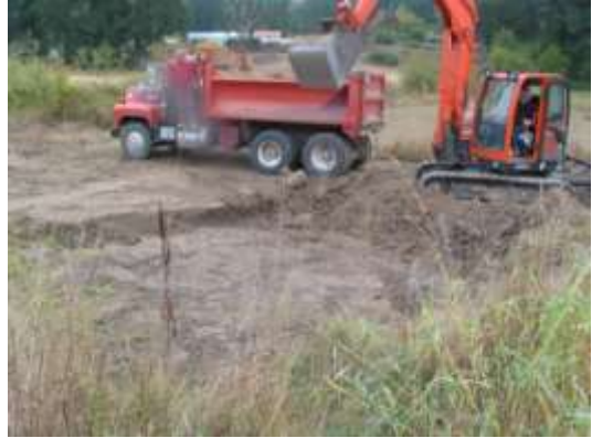
Implementation: An excavator creates the shallow pools adjacent to the existing pond.
