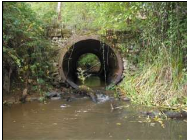
Before the project: Undersized culvert on Owens Creek that will be replaced with a bridge to accommodate crossing vehicle and livestock traffic. Note that the culvert's outlet is perched above the stream, and its diameter is much smaller than the stream's winter width.
