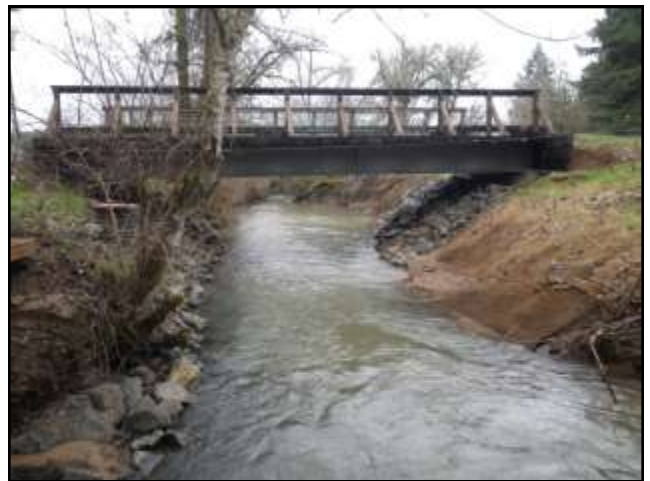
Implementation: This new bridge replaced the undersized culvert at Deck Family Farm.
