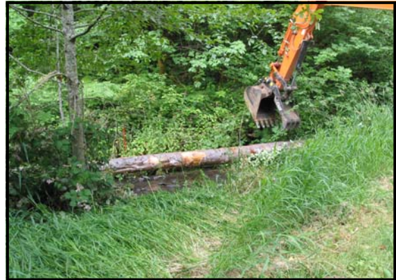
An excavator places a log in Ferguson Creek at Holzbauer's in August 2004.
