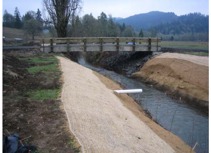
New bridge over Bear Creek. Banks were sloped back and covered with erosion fabric. Willows were planted along the edge of the channel and other native shrubs and trees higher on the banks.
