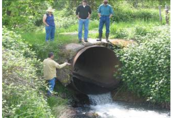
Pre-project: We removed this undersized culvert that blocked fish passage to 5 miles of essential cutthroat trout habitat.
