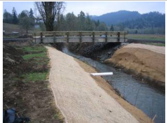
Post-project: We replaced the above culvert with this bridge that provides year-round cutthroat trout passage and decreased downstream erosion.
