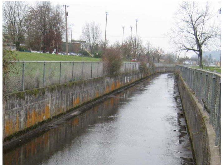
The section of Amazon Creek lined with concrete flows from about 24th to 16th street.
