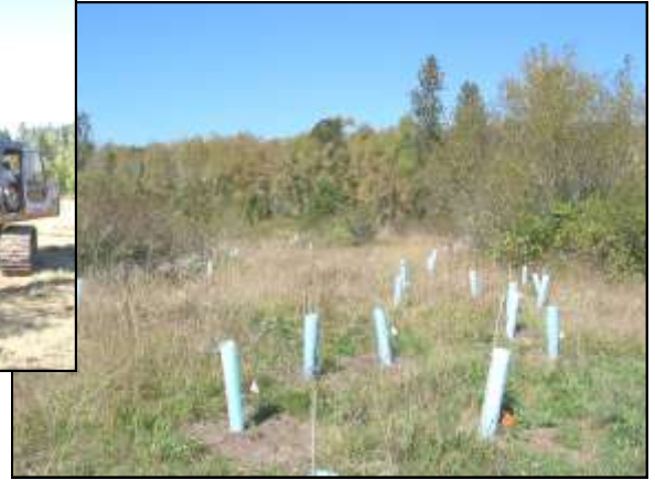
Top left: Engineers inspect a railcar bridge placed across a tributary to Spencer Creek on the Murphy property. Center: An excavator picks up a large conifer log to place in the stream Top Right: Oregon white oak, Nootka rose, and Pacific ninebark were among the trees & shrubs planted upslope from the creek.
