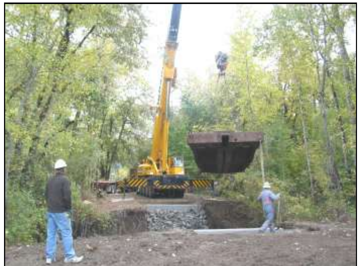
A crane places a railcar bridge over the tributary to Spencer Creek. This will allow the landowners maintenance access to the west side of the property.
