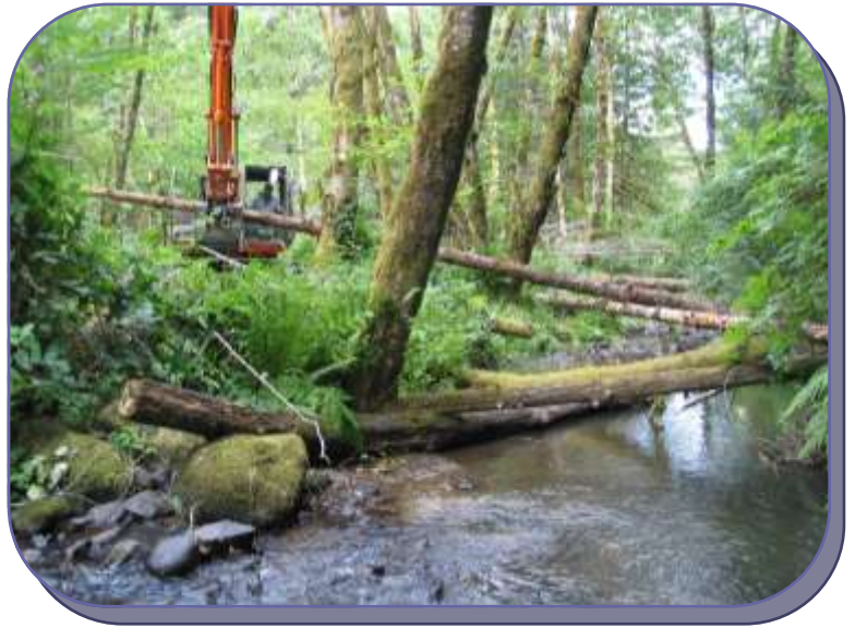
An excavator was used to place large wood at 5 sites along Ferguson Creek at the Holzbauer property.
