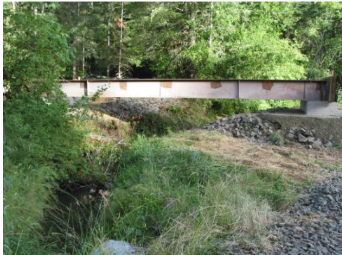
After the project: The undersized culvert was replaced with this bridge allowing year-round passage for cutthroat trout.
