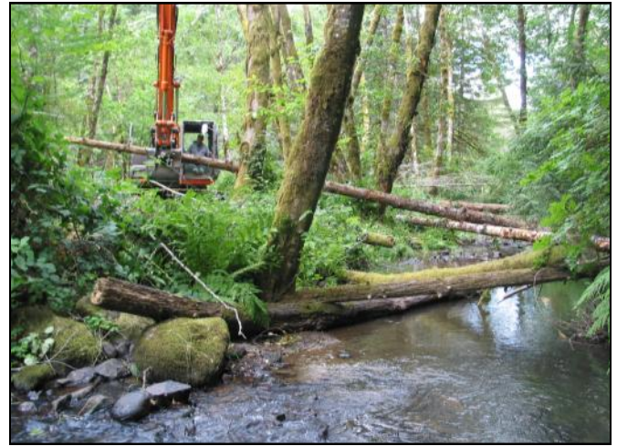
Implementation: An excavator was used to place large wood at 5 sites along Ferguson Creek.
