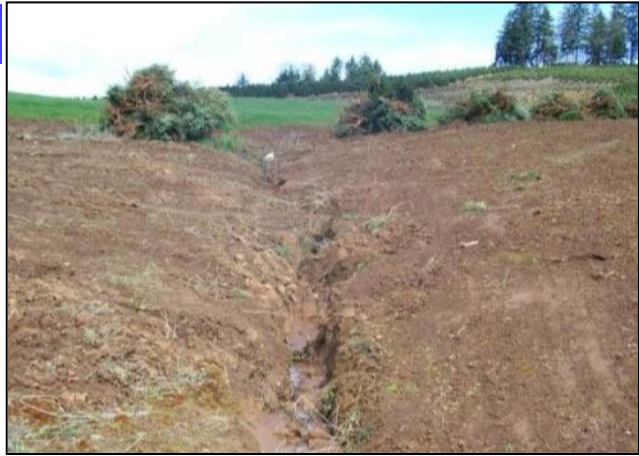
Pre-project: Photo shows bottom of drainage looking uphill. Note the lack of vegetation and deep gulying in the drainage channel.
