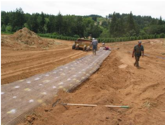
Implementation: The landowner uses a scraper and carry-all to construct the grassed waterway.
