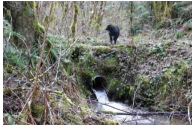
Before the project: This culvert was one of three on the Koehler property that were barriers to fish and amphibians attempting to migrate upstream.
