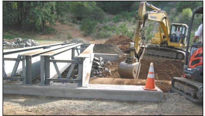
Bridge Construction: Support structure for bridge. Steel I-beams are connected to concrete footings set into the channel bank. Wood decking will be laid across the bridge. Rock rip rap is position at the base of the concrete footings.
