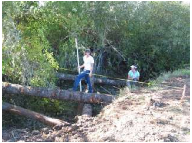
Implementation: Large conifer logs with rootwads were positioned in the tributary channel. In addition to enhancing habitat, these logs will help the channel's flow to naturally meander.
