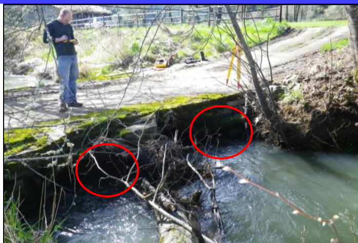
Before the Project: This crossing consisted of two undersized culverts on Ferguson Creek that created a velocity barrier for fish during most flows.
