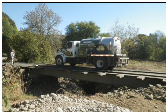
Implementation: With the new bridge in place, agricultural vehicles can now access the vineyard on the other side of the property, and native fish can swim upstream.
