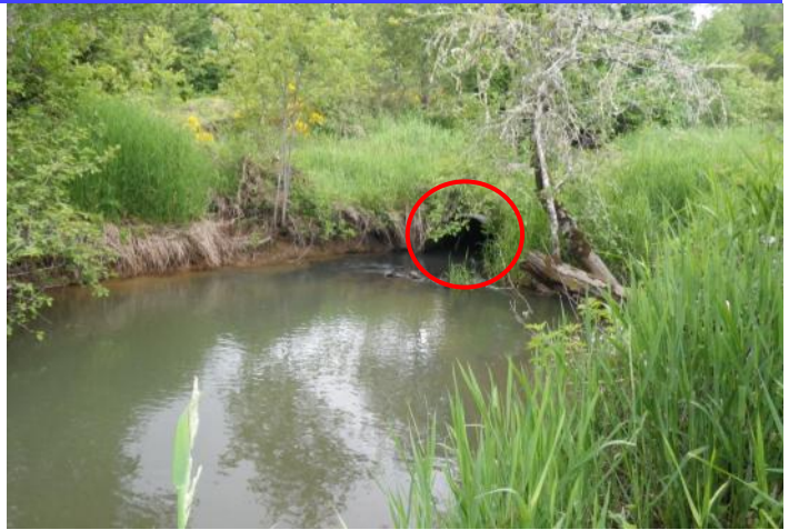
Before the Project: This undersized culvert on Owens Creek impaired fish passage during most flows.
