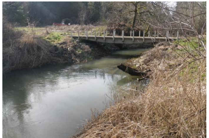
After the Project: The culvert was replaced with this 40' railcar bridge over Owens Creek.
