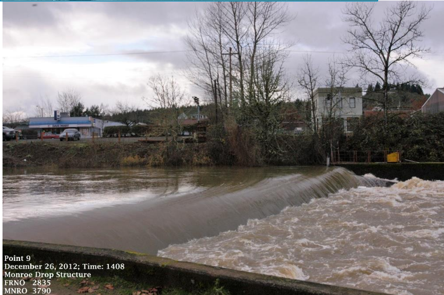
Figure 11. Monroe Drop Structure, looking west, at higher flows, Long Tom River, Monroe, Oregon
