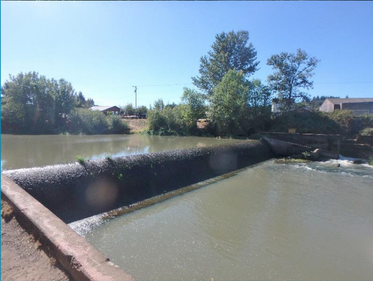
Figure 10. Monroe Drop Structure, looking west, at lower flows, Long Tom River, Monroe, Oregon
