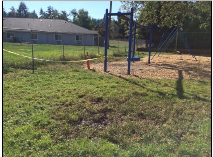
The playground at Ridgeline Montessori is soggy and muddy. Replacing part of the area with a constructed wetland will help divert water into the wetland, improving the playground and providing habitat.
