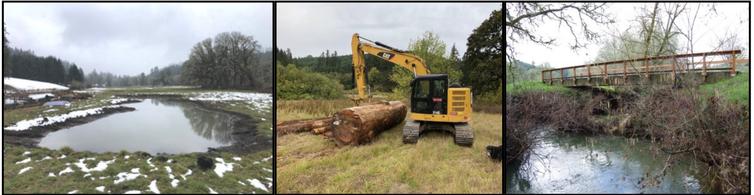
Photos from left: Melting snow in Feb. around one of the ponds created for turtle and amphibian habitat; a contractor prepares to push a piece of large wood into position; bridge over Bear Creek that replaced a culvert that previously blocked fish passage
