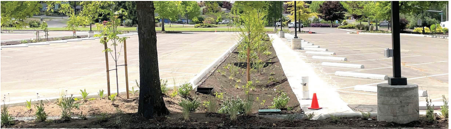
One of the four rain gardens installed at Willamette Christian Center. Visit longtom.org/wcctour2023 for more info!
