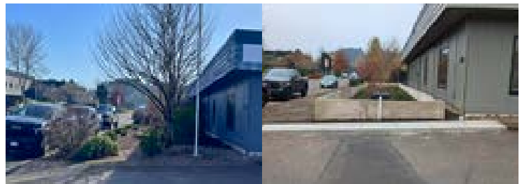
A BEFORE (LEFT IMAGE) AND AFTER (RIGHT IMAGE) COMPARISON OF THE GIBSON STEEL PLANTER. THE AFTER PICTURE WAS TAKEN APPROXIMATELY A MONTH AFTER INSTALLATION.
