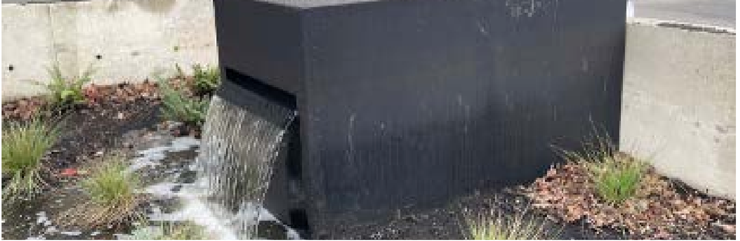
CUSTOM MODIFIED GIBSON STEEL SAND COLLECTOR BASIN, WORKING AS A SEDIMENT DROP FOR THE NEW PLANTER INSTALLATION.
